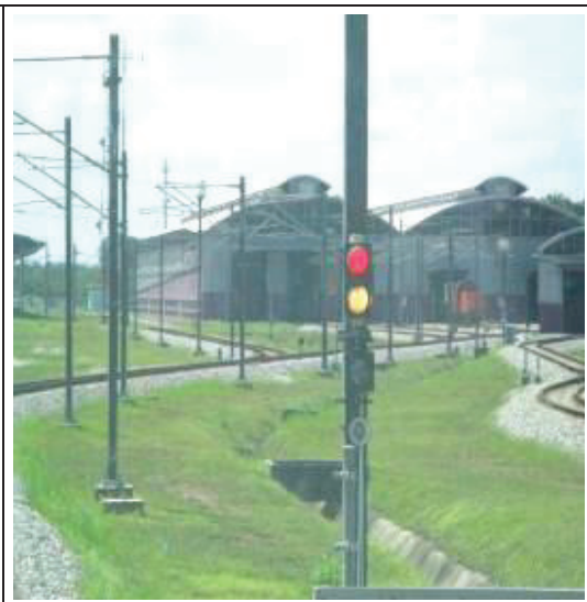
Pic 2 - Positioning Signal Flashing RED & WHITE
