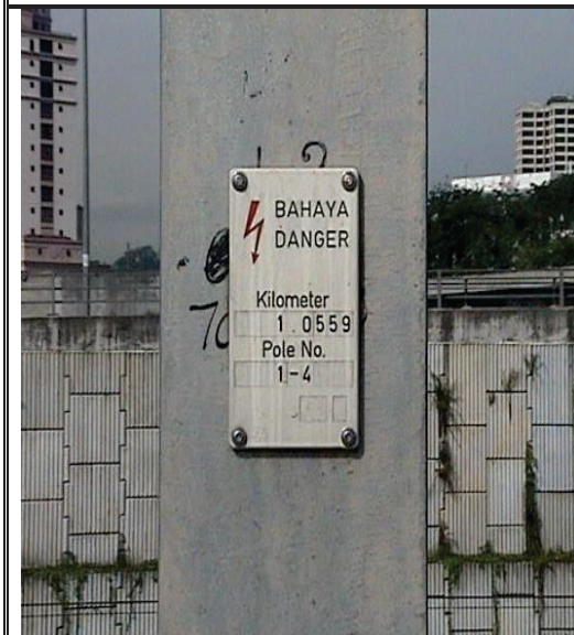
Figure 3: Chainage marker (small white plat) stated the actual position (KM), which to be used for keying-in the position on the ATP MMI.
