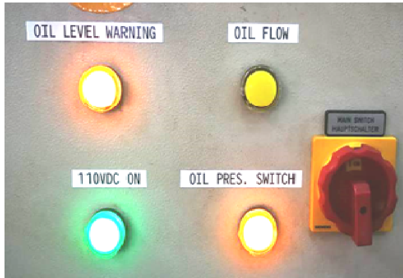
Figure 12.4: Oil Flow indicator de-illuminated
