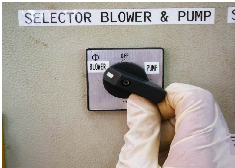
Figure 12.9: Selector Blower & Pump
